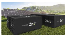
Zinc-air flow batteries
