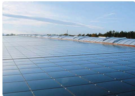
Thuringen, Germany 340 kWdc
