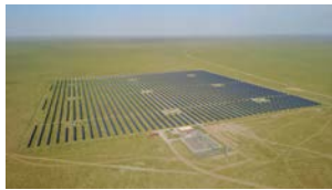
Industrial Solar Power System
