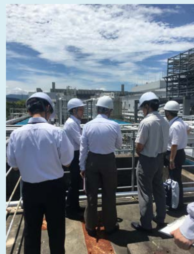
RBA auditor (third from left) checks factory wastewater treatment equipment together with Sharp personnel
