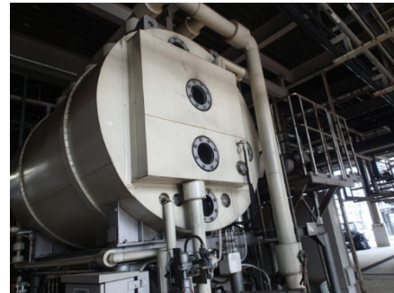
Evaporating and concentrating a portion of washing waste liquid at an on-site facility
