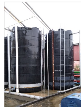
Rainwater tanks installed in the plant
